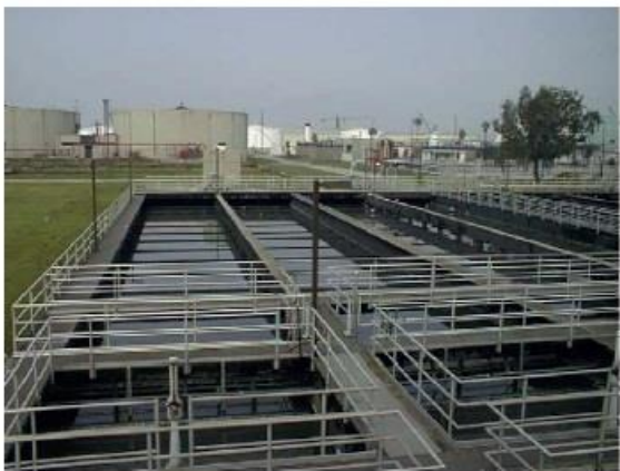
Figure 7.7 Rectangular primary clarifiers.
